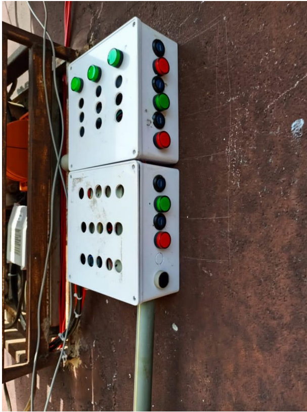
Figure 25 - Image of the new central control unit.
