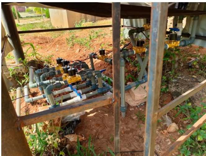
Figure 24 - the valves set up
