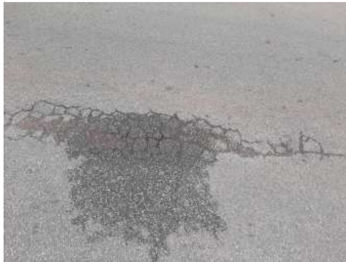
Plate 2: Medium severity Alligator crack along the road
