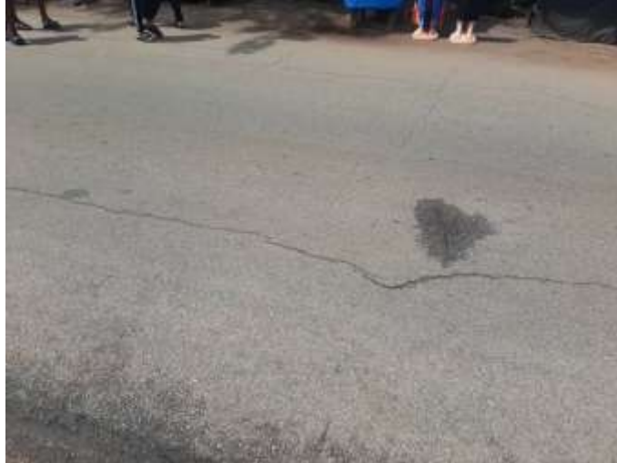
Plate 3: Low severity Longitudinal crack
