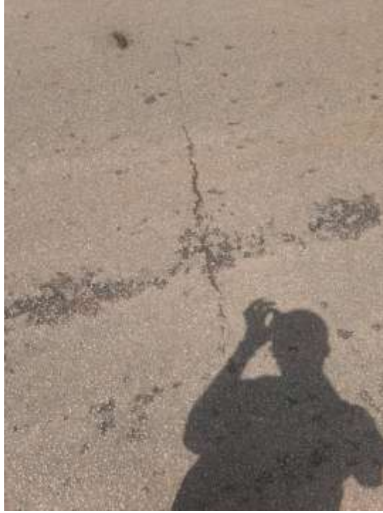
Plate 5: Low severity Transverse crack
