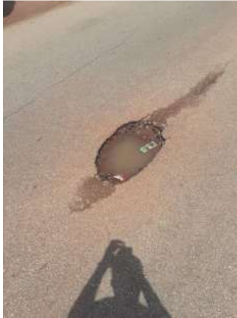
Plate 1: High severity Pothole in the study area
