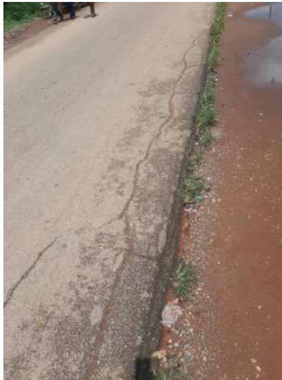
Plate 4: Medium severity Edge Crack
