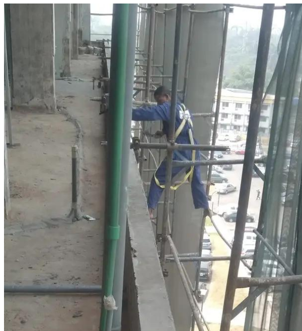
Figure 4.5: A view of the unclad frame structure of Block B during the renovation. (Source: Field work 2022)
