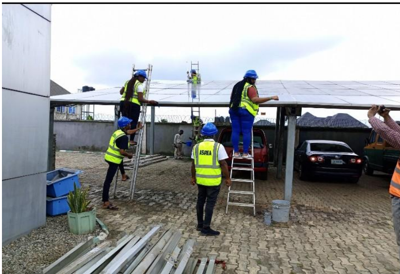
Sourced from field work showing maintenance of a solar panel and a closer look on the panel.
