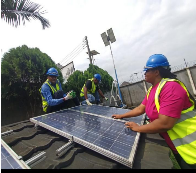
sourced from field work , showing how panels are arranged in arrays
