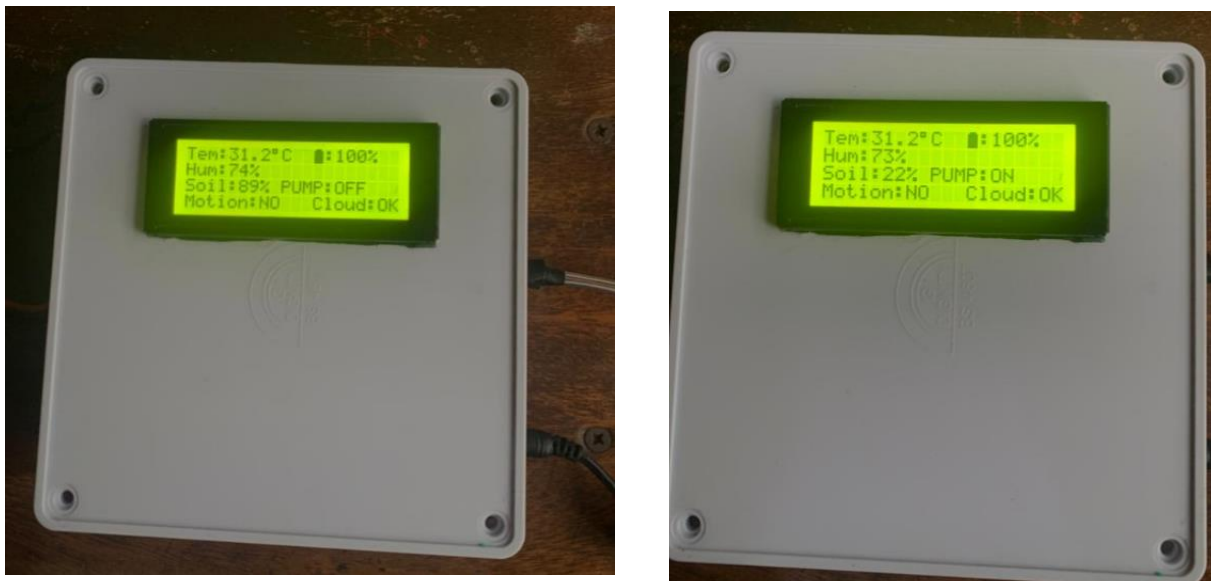
Figure 4.3: LCD showing the Pump off and on based on the threshold values
