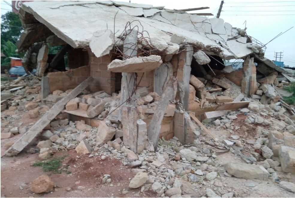
Plate A-3: Building after collapse
