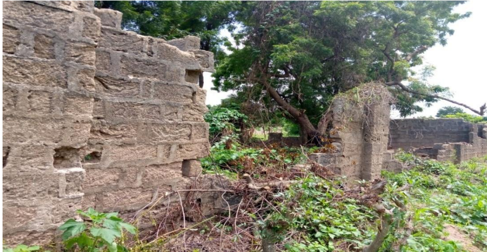
Plate E-3: Building after collapse
