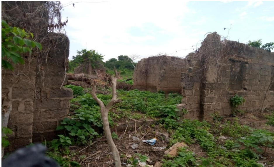
Plate C-3: Building after collapse
