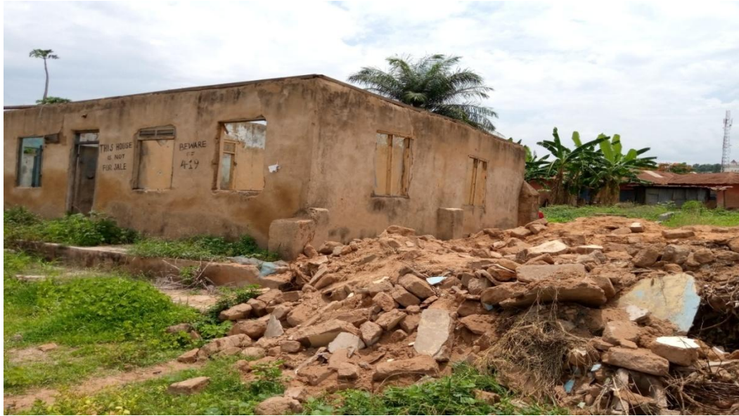
Plate D-3: Building after collapse
