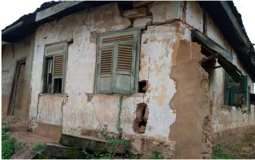
Plate B-3: Building after collapse
