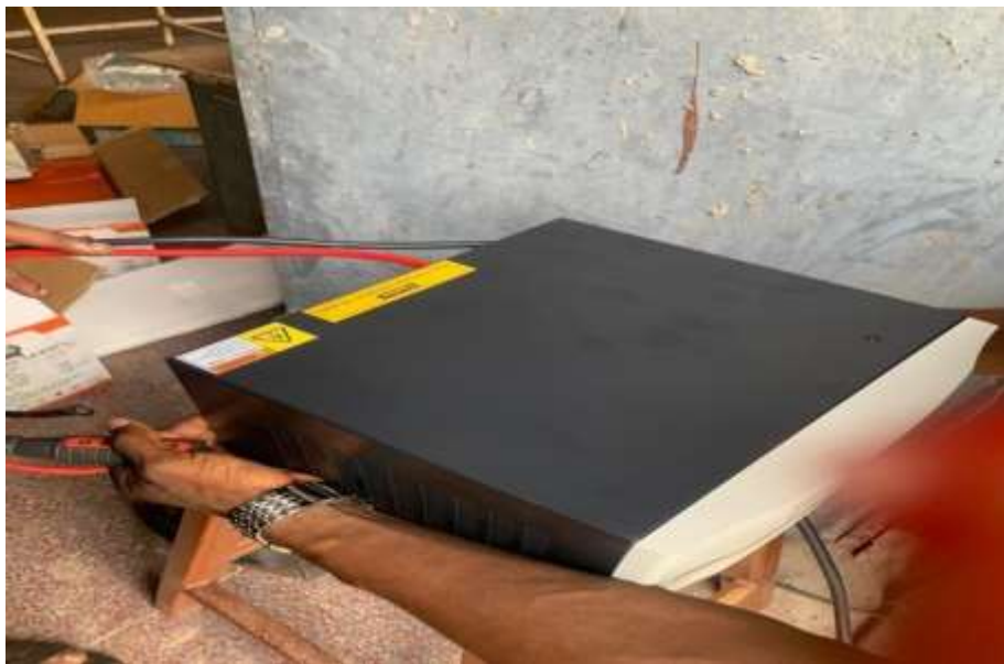
Figure 4.7: Inverter system connection
