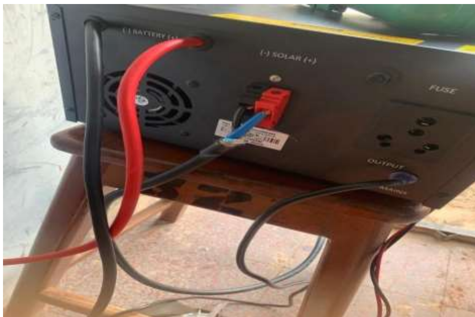
Figure 4.9: Rear view of the inverter showing connection of the battery, PV array and output.
