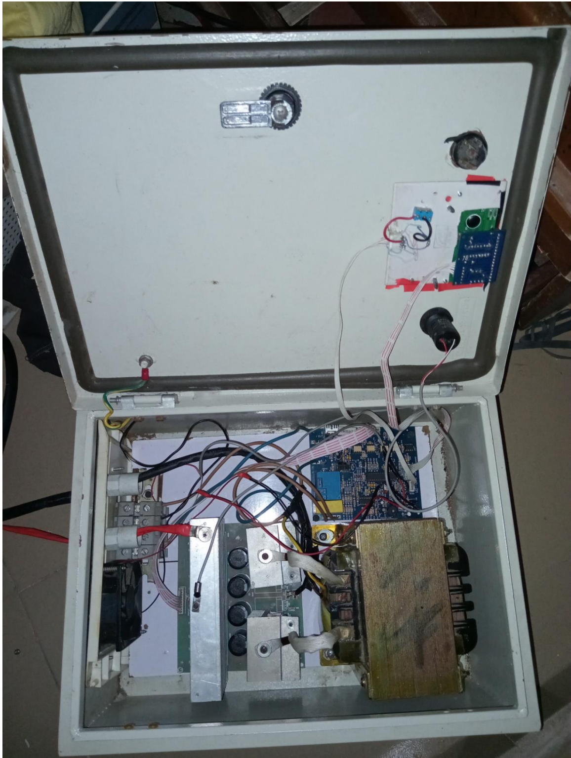
Figure 4. 13: Internal View of Inverter Package
