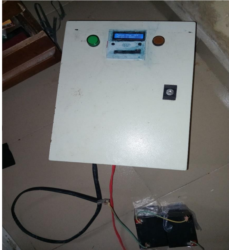
Figure 4. 15: Testing the Inverter
