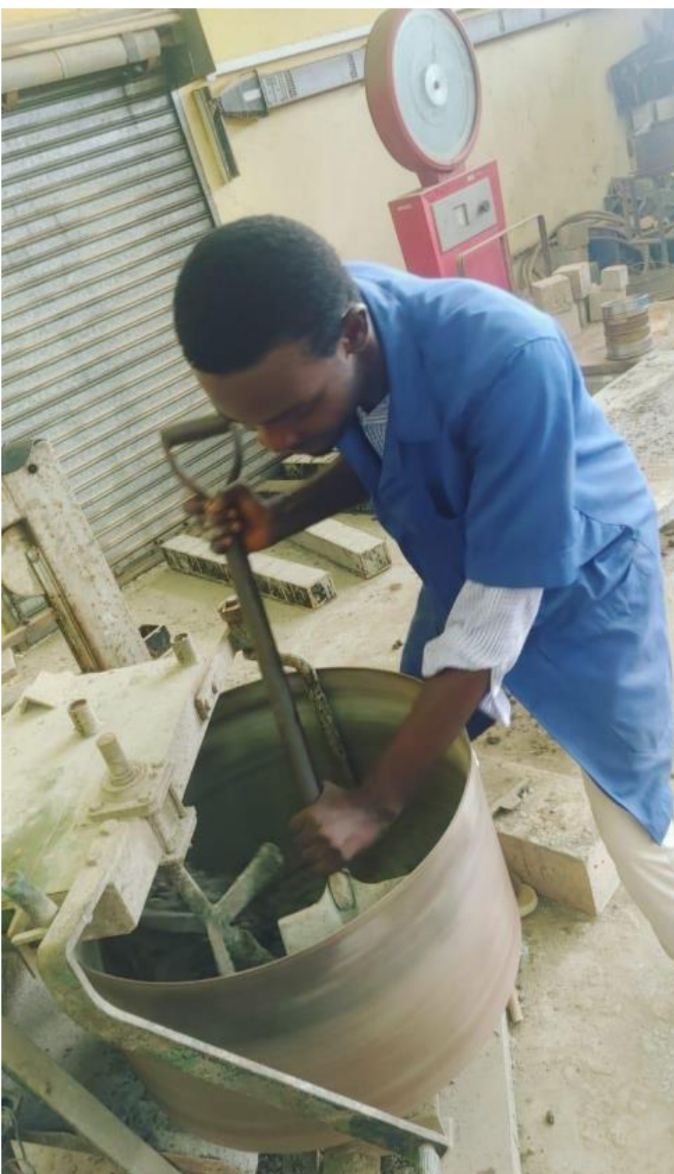
Plate D4: Mechanical mixing of concrete constituents using a rotary drum mixer
