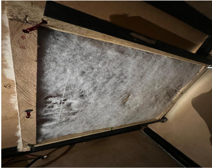
Figure 3.6 Wood insulated for extractor hood
