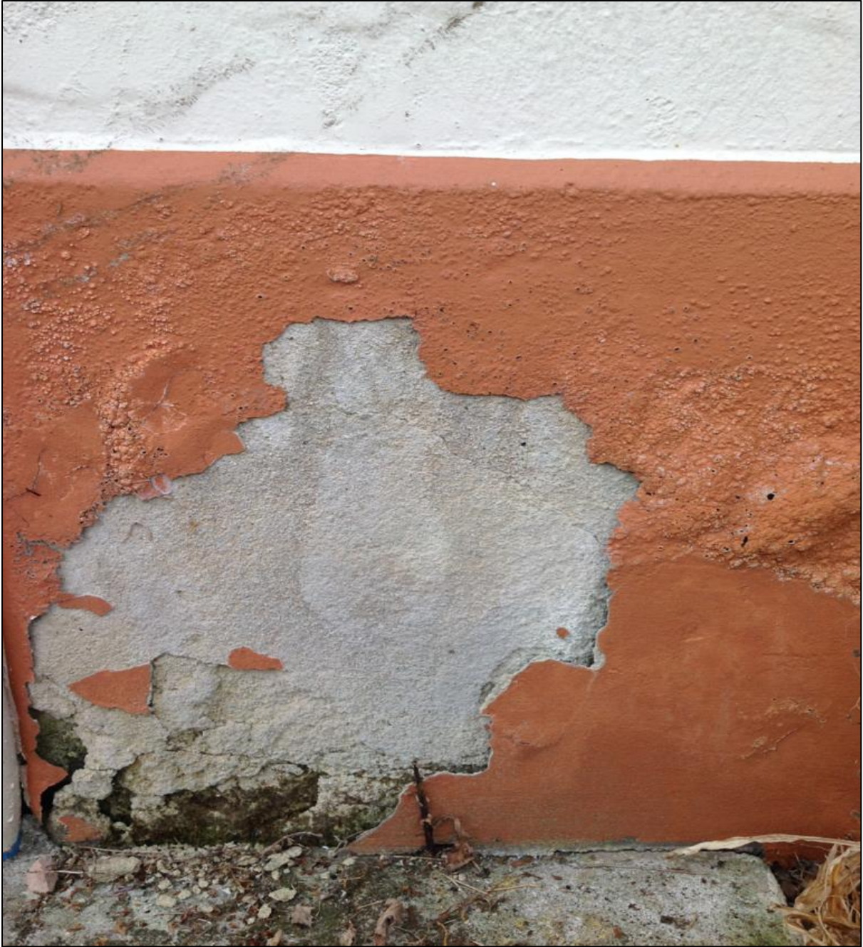
Plate 1: Deteriorated emulsion-painted wall.
