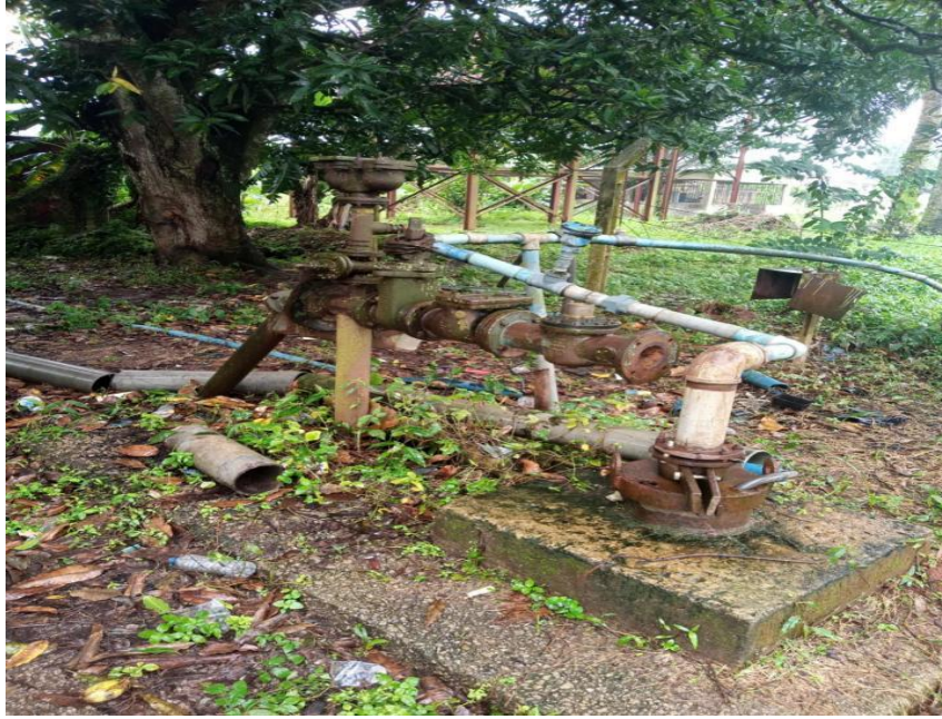
Figure 3.2: pump at the Uniben Water Scheme
