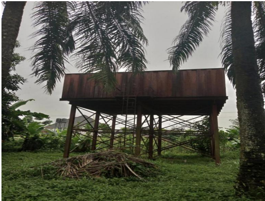
Figure 3.3: Overhead Steel Tank at the Uniben Water Scheme
