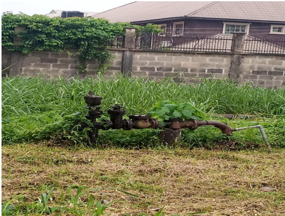
Figure 3.5: Valve at the Uniben Water Scheme
