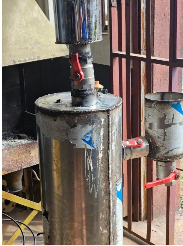
Figure 4.7: Slurry Valves on the Canister System
