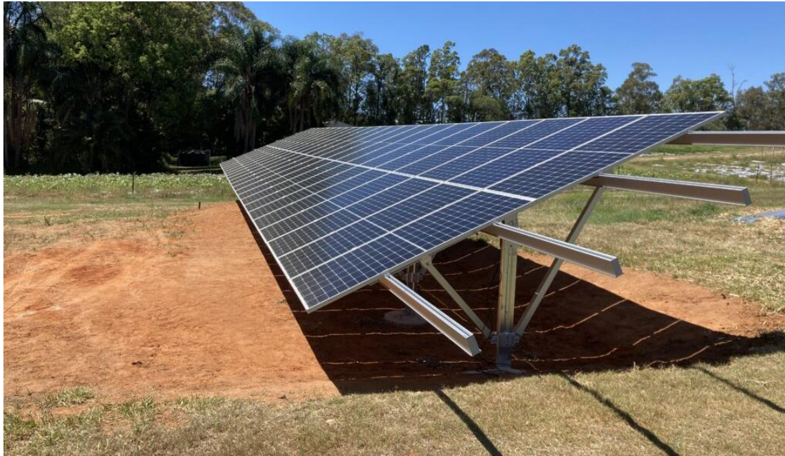
Figure 4.2: Solar panel mounting structure
