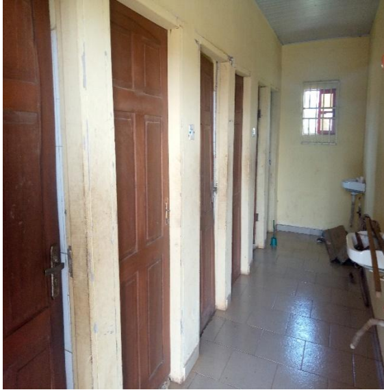
Plate 3.5: Non- functioning hand washing basins at Uselu market
