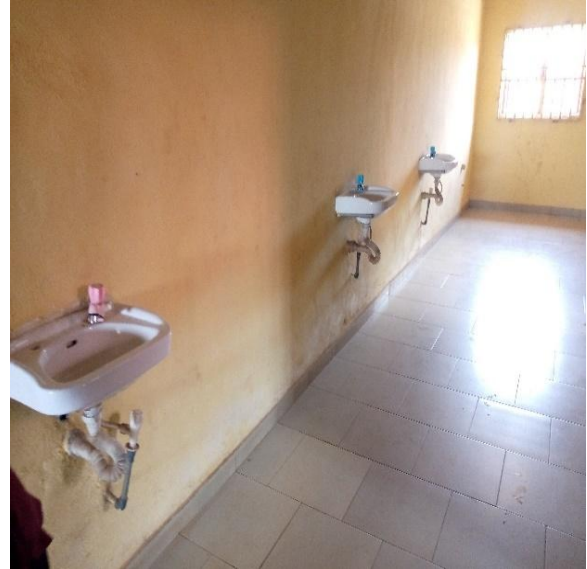
Plate 3.10: Nonfunctioning hand washing stations at Ogida market
