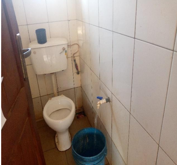
Plate 3.9: Flush toilet at Ogida toilet facility
