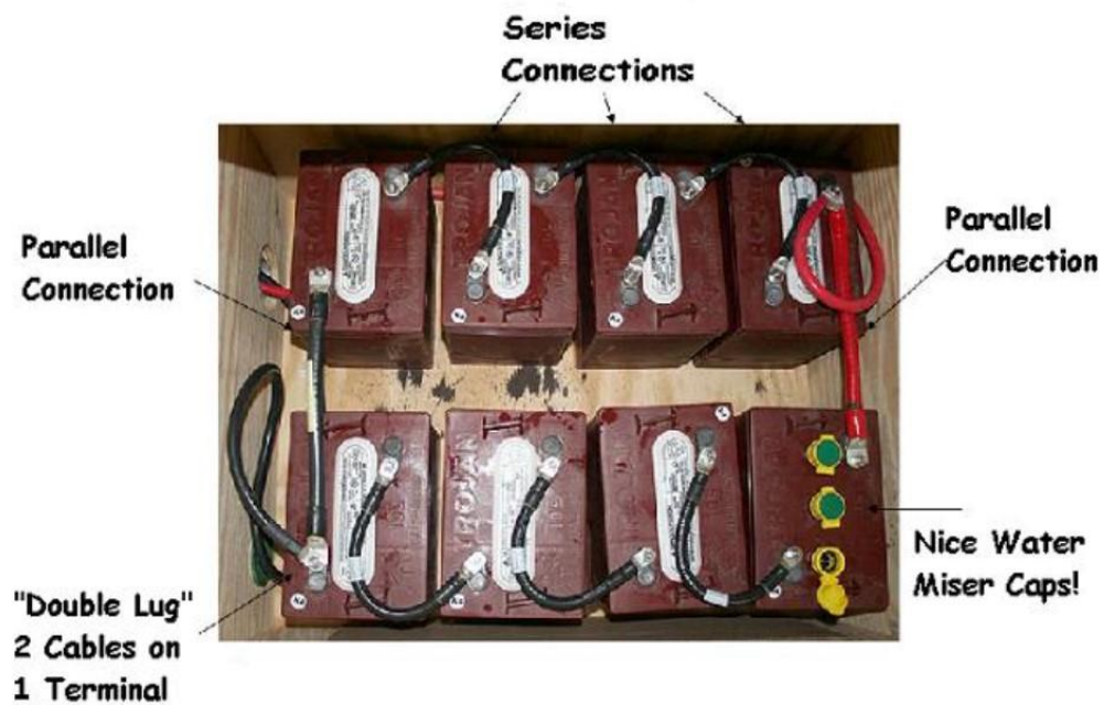
3.2: Battery Arrangement and connection (altE)
