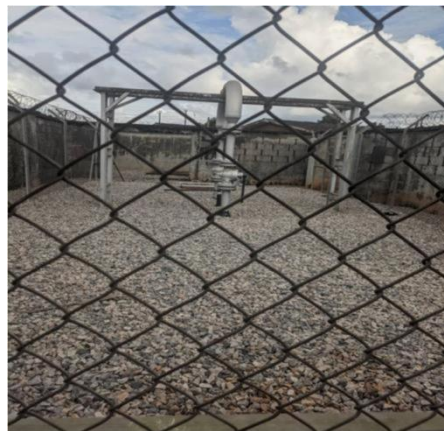
Figure 3.4 Above ground metering station
