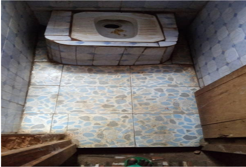
Plate 4.1: A toilet with Indian toilet seat in a bad condition.
