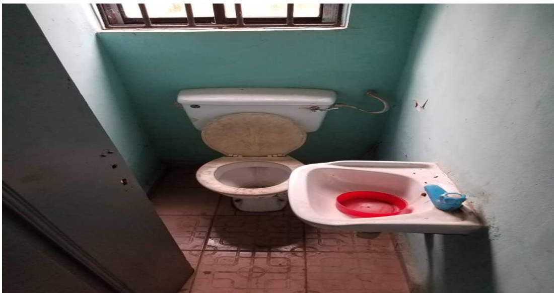
Plate 4.3: A poor state of toilet in the study area
