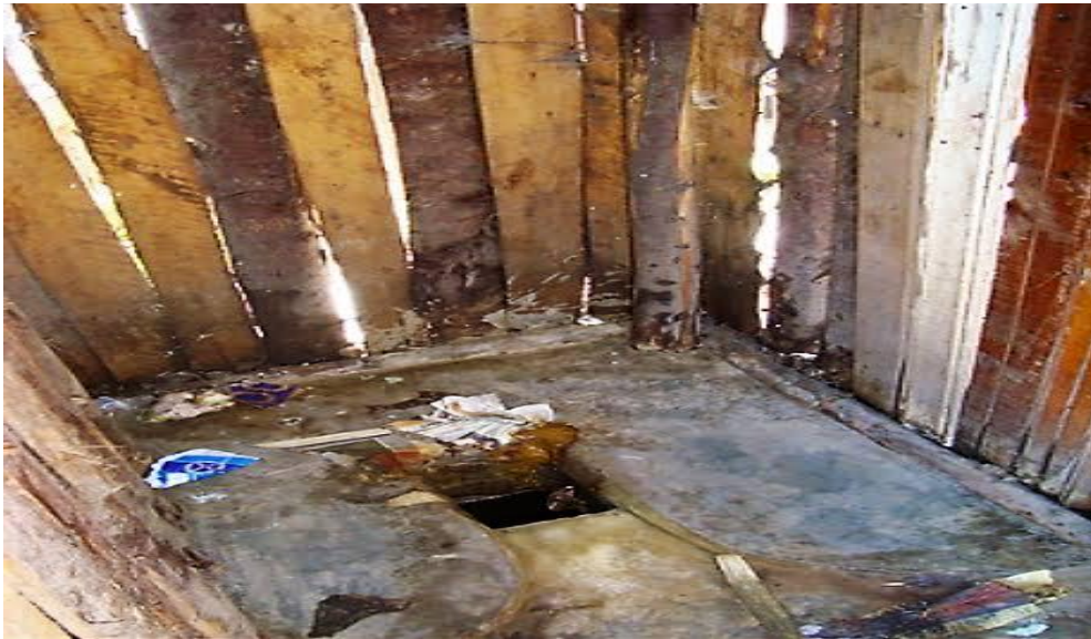
Plate 4.2: A pit toilet in bad condition.
