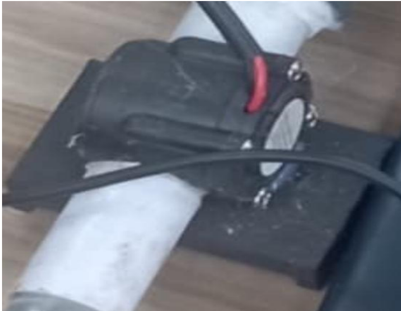
Fig 4.2.3. Working on the SF-Y201 Flow Sensor
