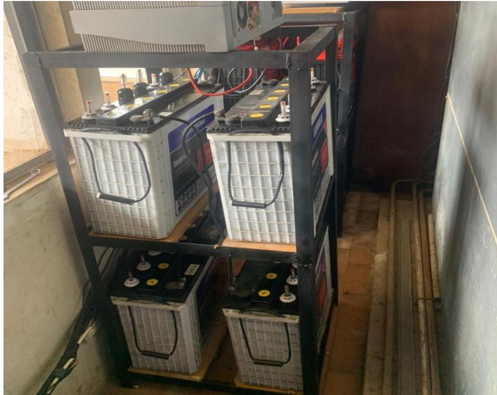
Fig 7: showing the arrangement of batteries in frame
