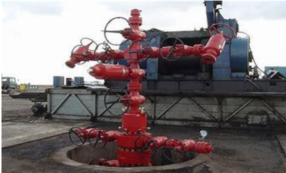
Figure 1.1 christmas tree installed on offshore platform
