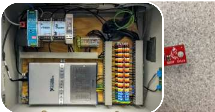
Figure 3.13 a) DAQ system (Akita et al., 2020) b) Downhole inclination sensor
