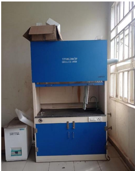
Figure 2.13 The university of Benin central laboratory fume cupboard
